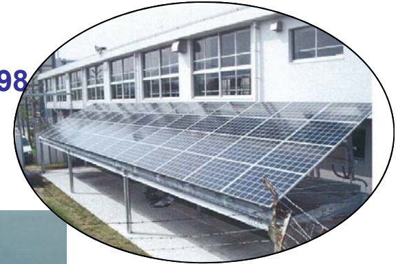
R&D on recycling technologies for solar power systems
